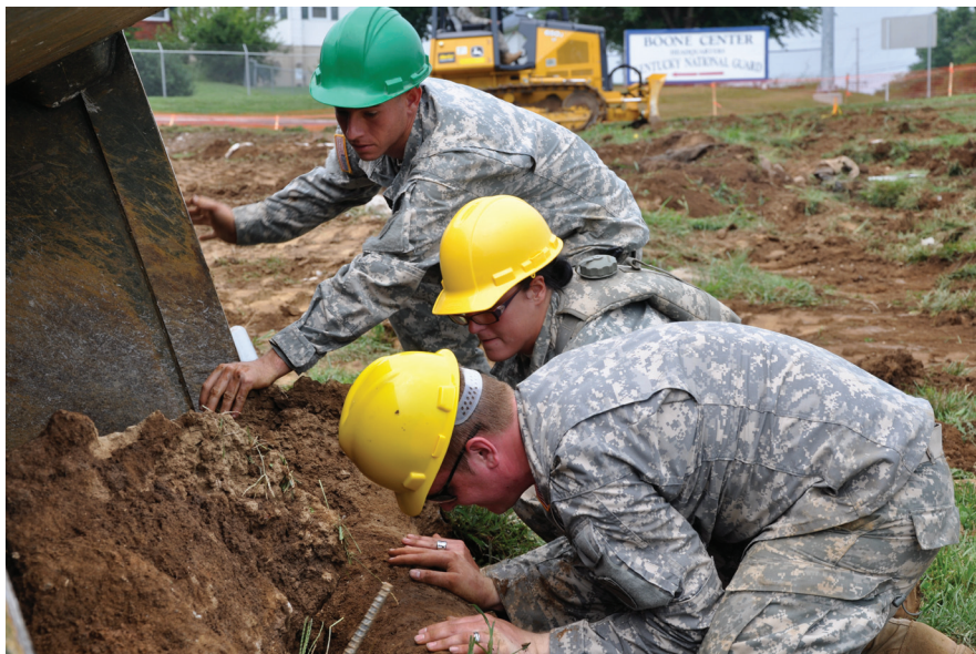
Pvt. John Law, 130th Engineer Support Company, 206th Engineer Battalion signals to the dozer operator as Spc. Sarah Setser and Spc. Joshua Smith of the 207th Horizontal Engineer Construction Company, 201st Engineer Bn., push rubble into the bucket.
